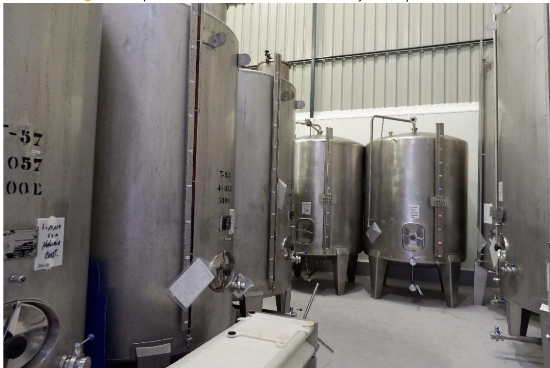
Figure 5 - Aspect of the estufa room of the MWC winery at Caniçal. 19-12-2019
